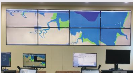
VTMS Control Room
